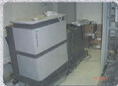
Hi-Path 4000 Server at Data Center
