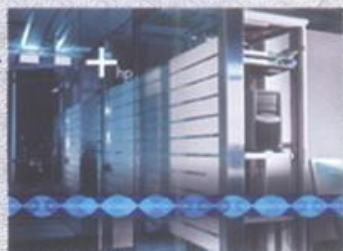
HP Pro-Liant Servers are used in the data center to provide unprecedented support.
