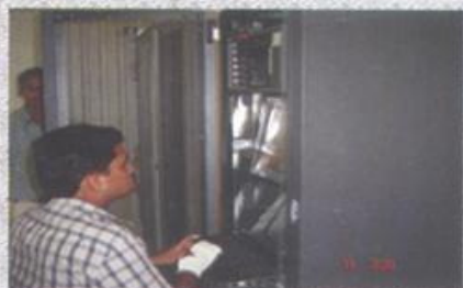
Project Engineer M. Sadiq Ali Khan configuring the wireless bridge at the Data Center.
