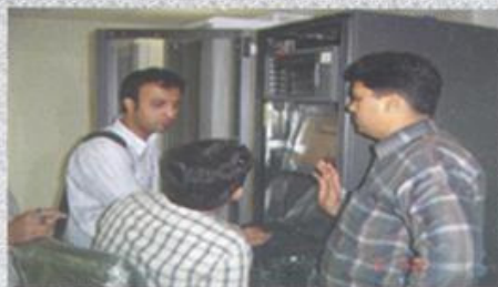
Server Configuration at Full Throttle at the Data Center of High Speed Fiber Optic Based Network.
